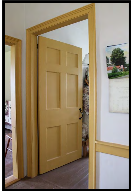
Figure 81: Reconstructed Door, Norfleet House.
