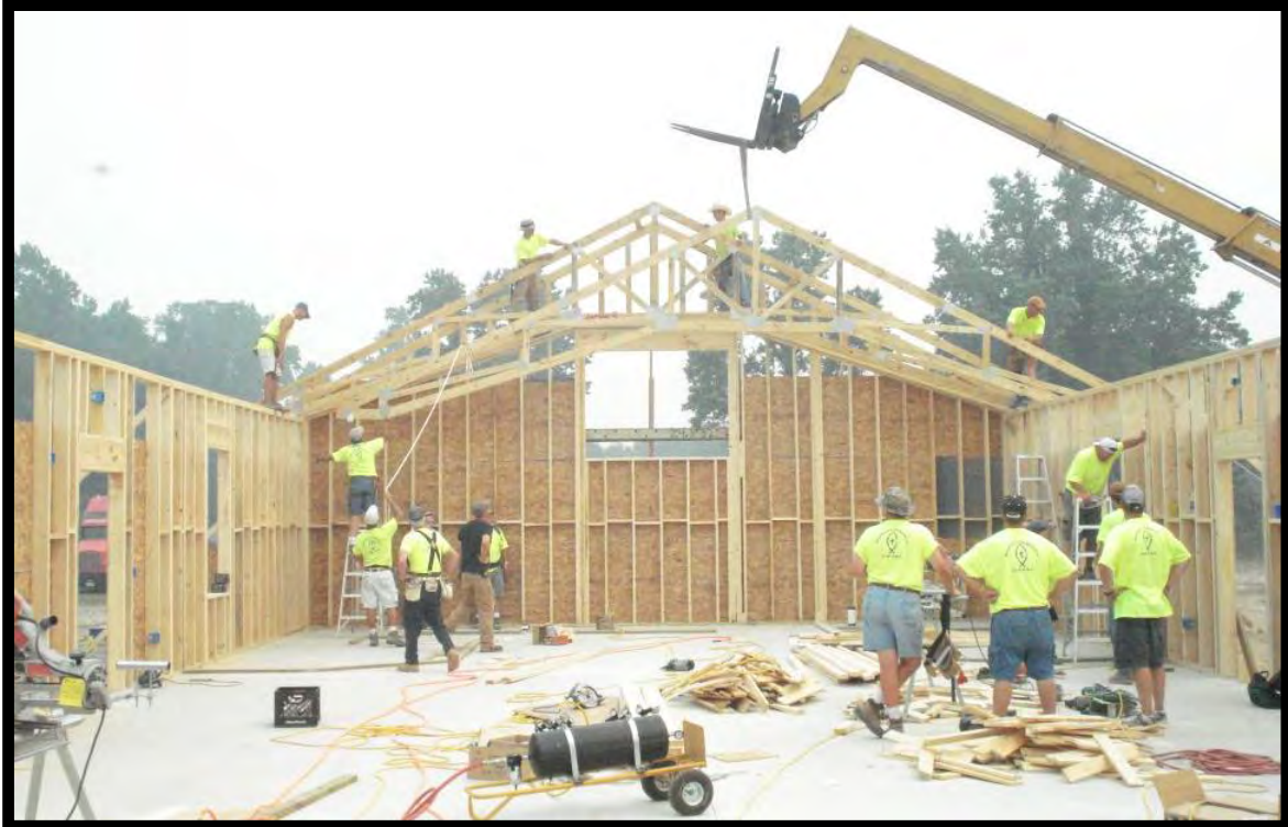
Figure 65: Volunteers from Meshach's Carpenters Placing the Trusses of the New St. Paul AME Zion Church (Meshach's Carpenters Facebook Page).
