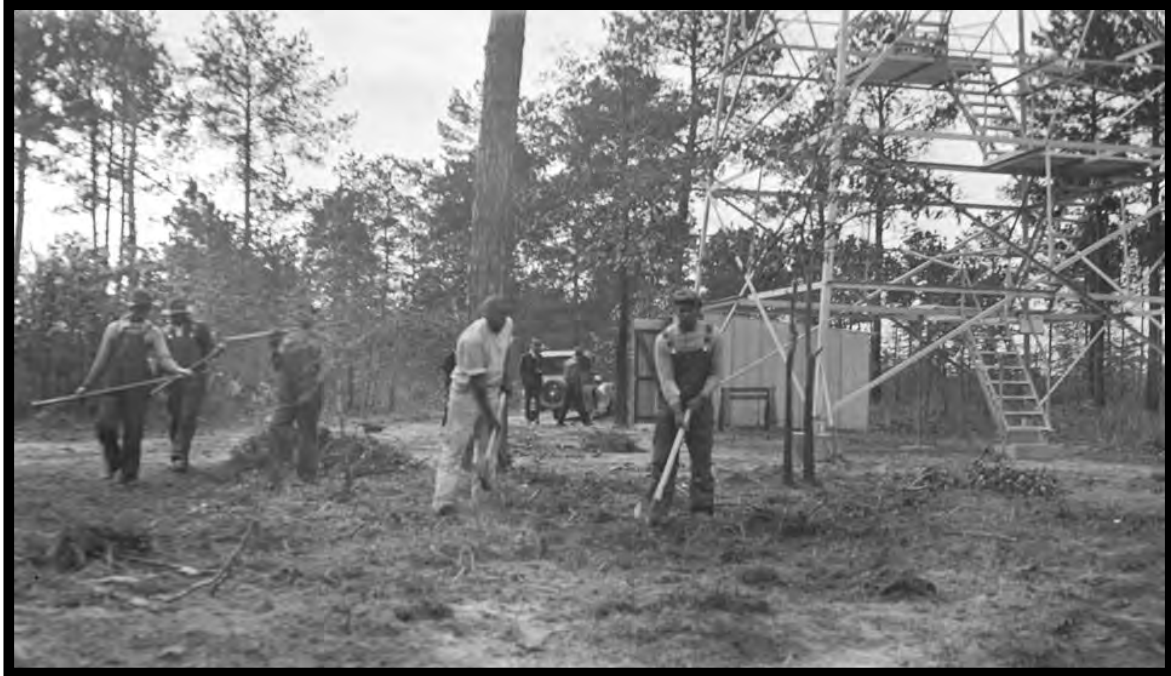
Figure 106: “Improvements - fire lookout tower. With use of unemployed serving as a fire crew. Edgecombe County, North Carolina.” (Forest History Society, Durham, N.C.)
